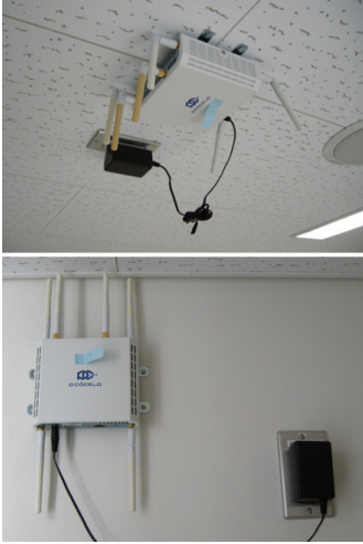
Fig. 5. PCWLs installed on the ceiling and the wall.
